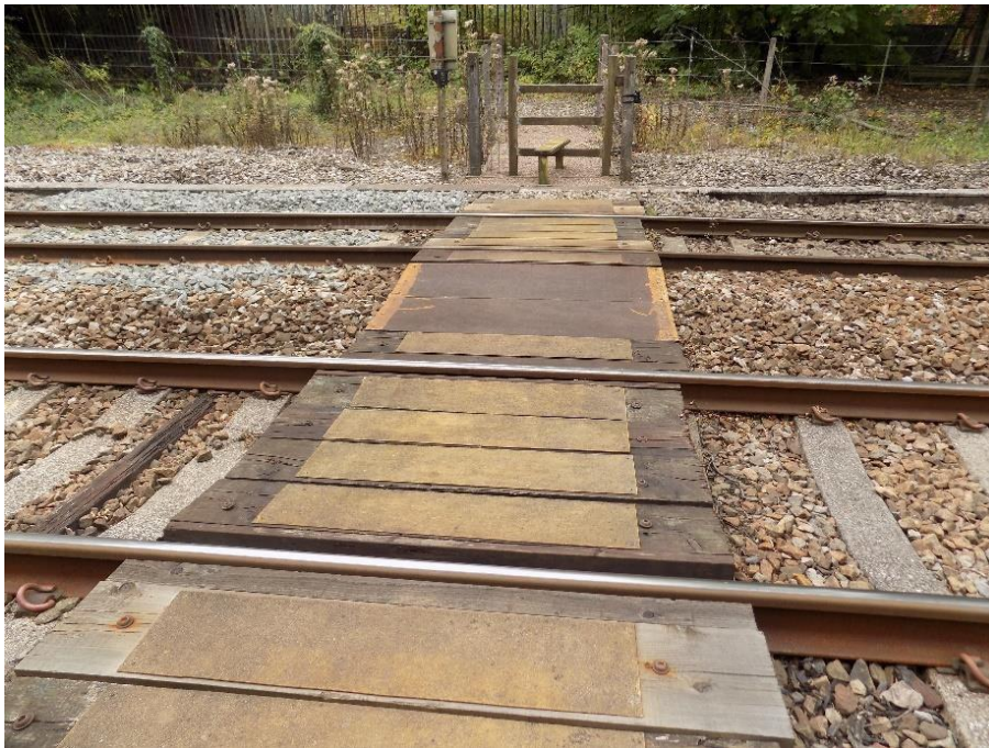
Figure 2-4.8: Level crossing deck
